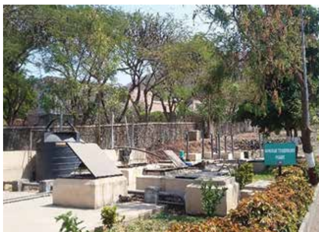
Sewage treatment plant
